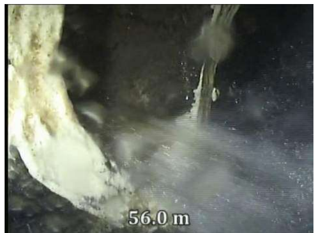
Figure 6: CCTV Report Extreme Inflow Noted at Main St and St. John
